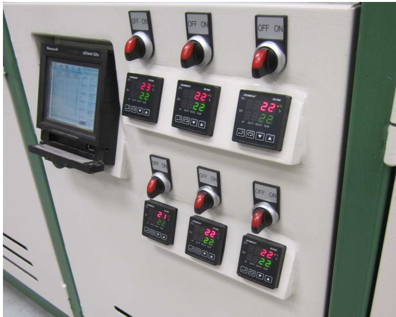
Figure 2: MFA Temperature Controller Cabinet
