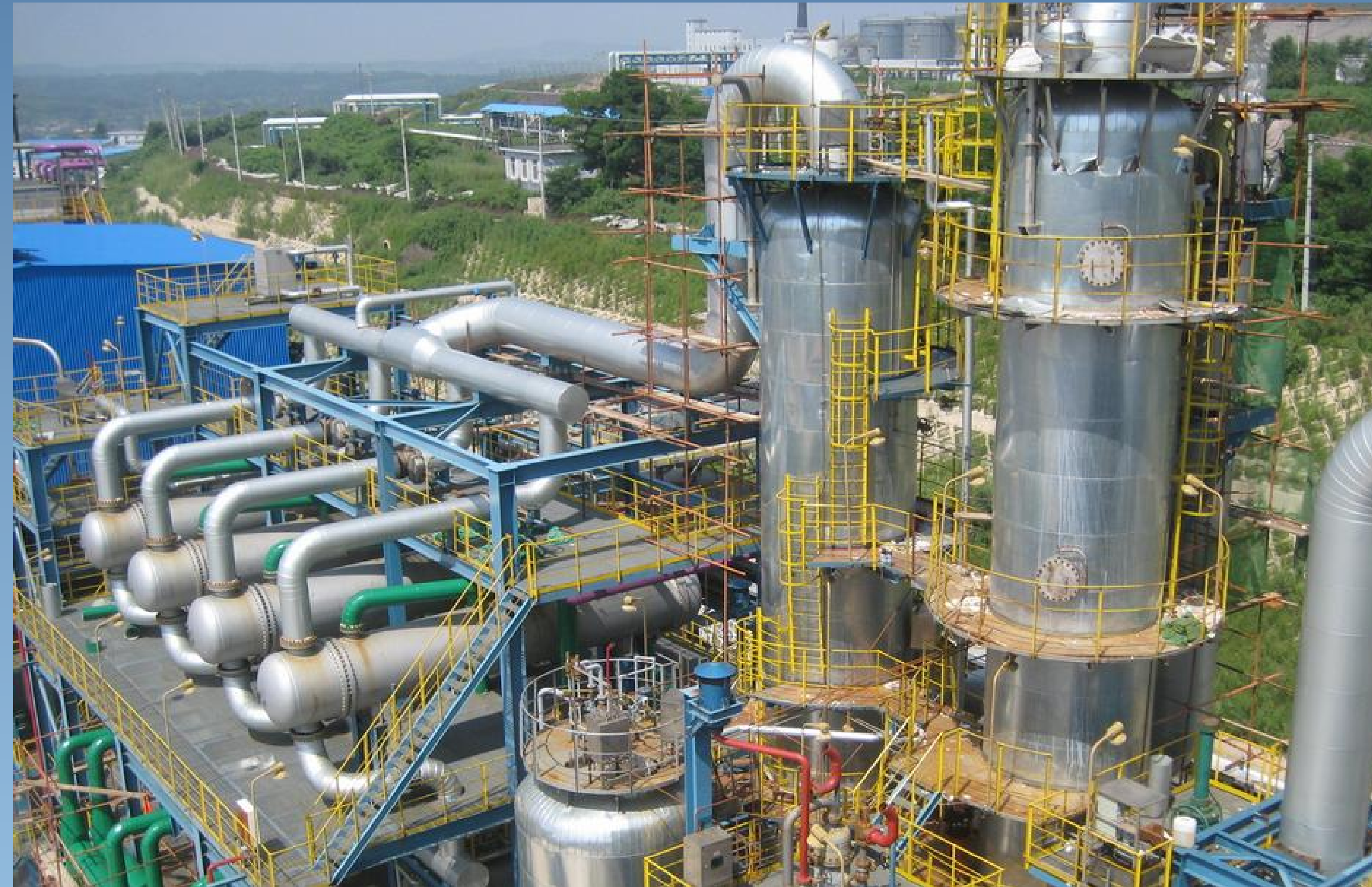
Above: The Oil Recovery System
